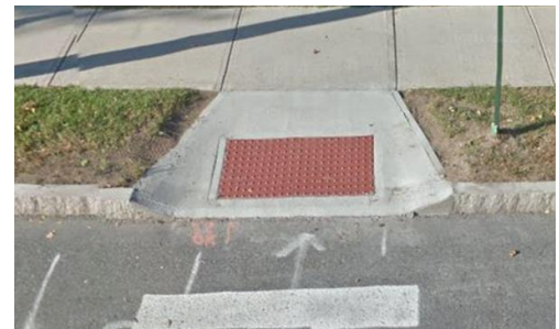
Figure 2 Grade breaks and edges of a ramp should not be rounded, as shown here
